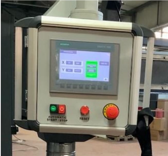
Touch Panel Siemens
